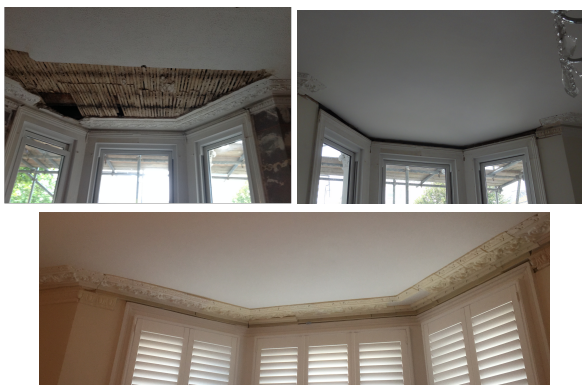
Figure 1: Ornamental moulding in need of restoration in the interior of a household; top left) initial state of the ceiling; top right) ceiling after restoration with no ornament; bottom) restored area before gluing the ornaments to the ceiling and painting them
